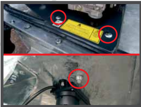
ANTI-THEFT BOLTS SECURING THE PRESSURE WASHER TO THE CHASSIS
